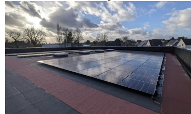
LANVALLAY 74 KWc Centre Technique Municipal
